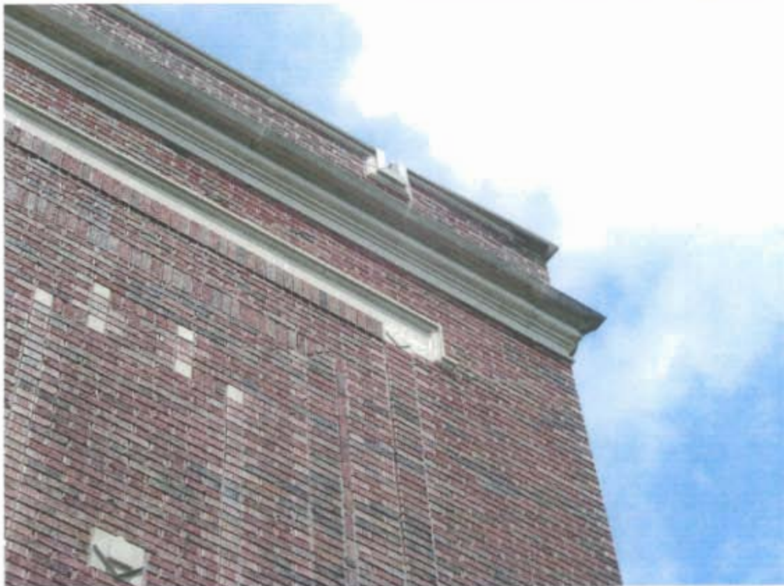
Photo #8: Southeast corner of building showing missing capstone at roof parapet. Metal roof cap was installed without replacement of stone cap.
