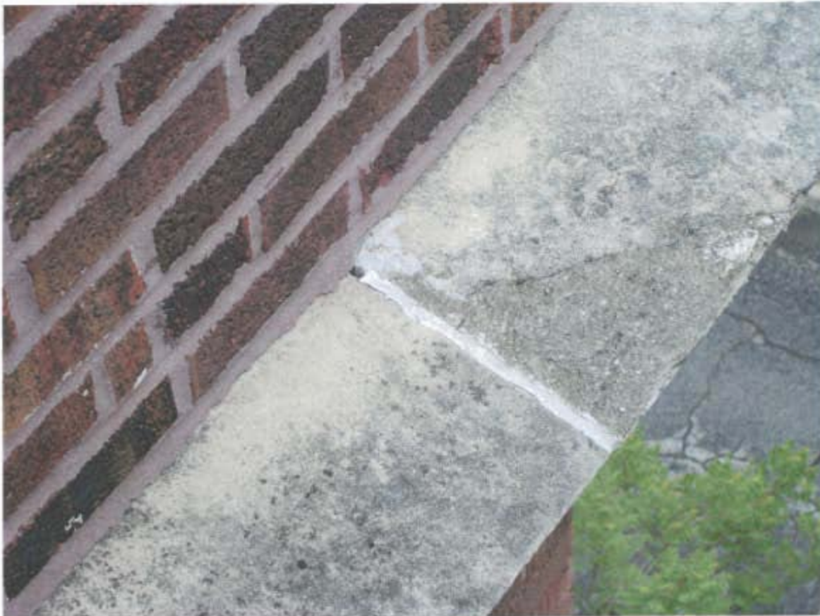
Photo #12: Failing caulk joint at perimeter stone band.
