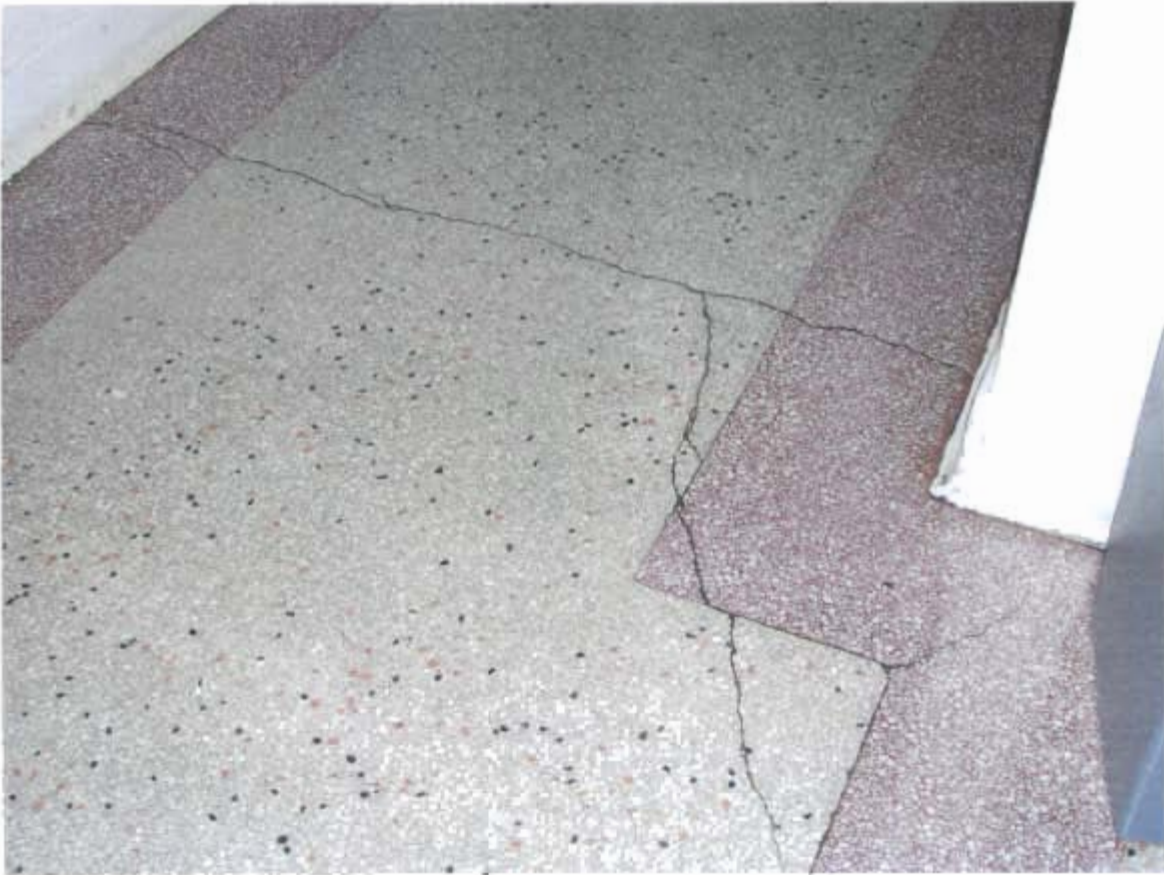
Photo #1: Random cracking in terrazzo floor at first floor near north stair.
