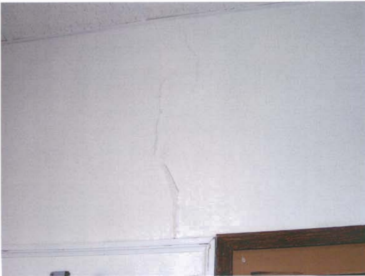
Photo #3: Vertical crack in plaster at first floor east corridor wall at south end. This occurs at this location at each floor.
