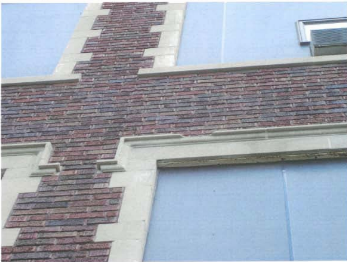
Photo #20: Damage to stone window header at east wall, second floor.
