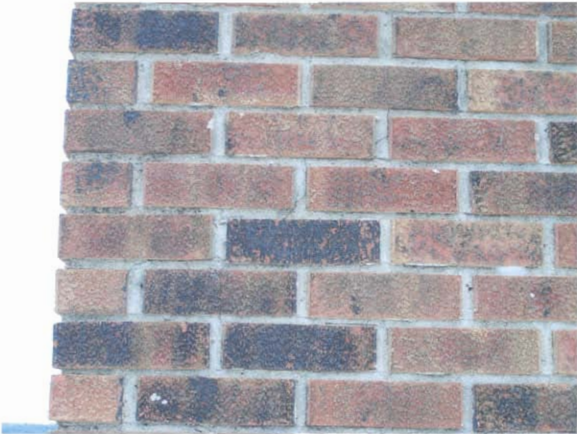
Photo #13: Diagonal crack in masonry veneer at west chimney.
