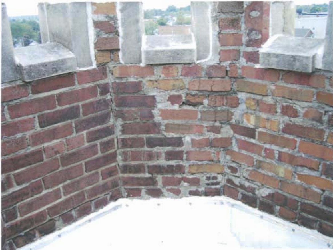
Photo #10: Failing mortar joints at inside face of front entry tower (above roof).
