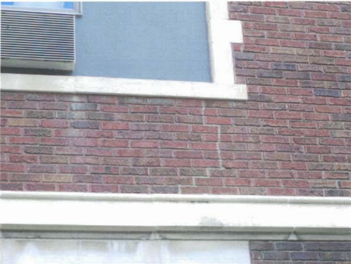
Photo #16: Previously repaired crack below second floor window.
