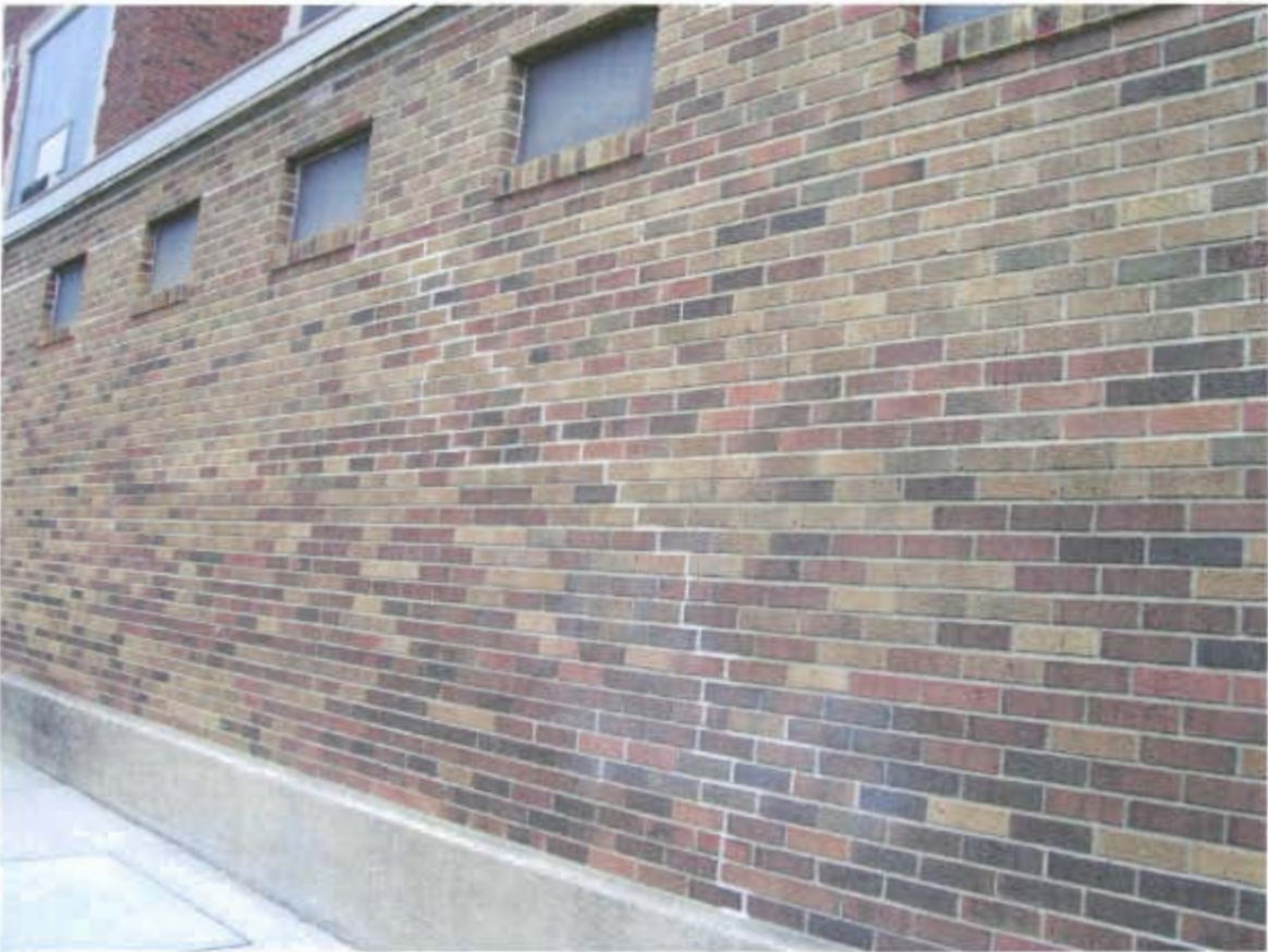
Photo #14: Previously repaired masonry crack at first floor locker rooms (now storage) at west wall.
