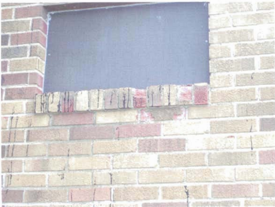
Photo #19: Brick spalling at north wall of locker rooms (now storage).
