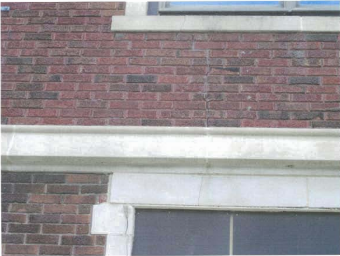
Photo #21: Crack in stone and masonry on east wall near south end. First floor window head to second floor sill.
