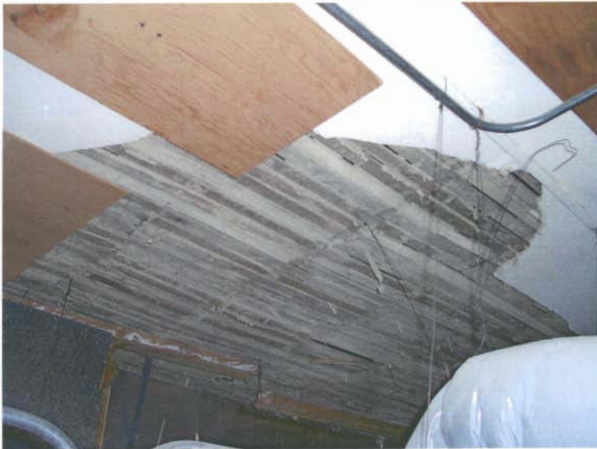
Photo #4: Falling plaster at first floor classroom ceiling (across from Library). Wood lath and plaster on 2x wood framing.
