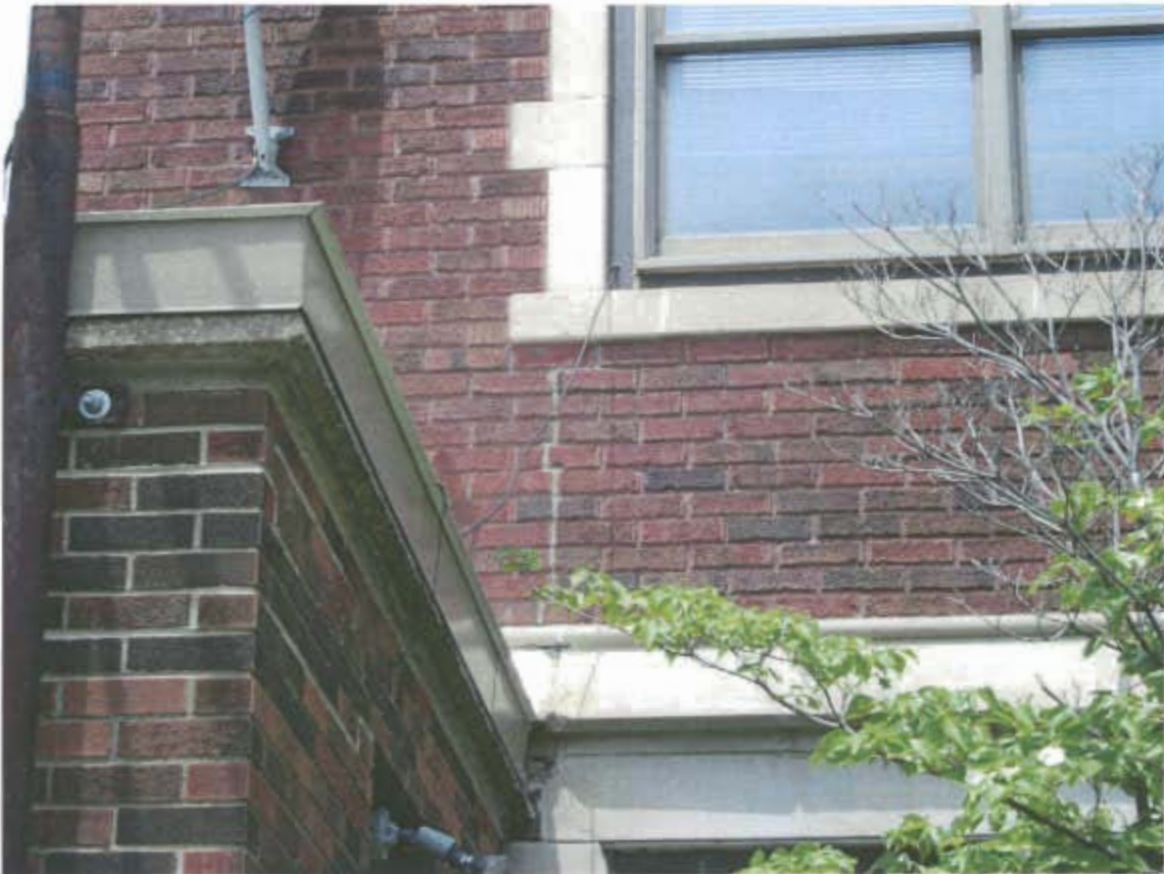
Photo #18: Previously repaired masonry crack at south wall, first to second floor.
