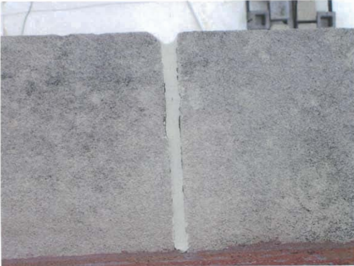
Photo #11: Failing caulk joint at stone band just below parapet.
