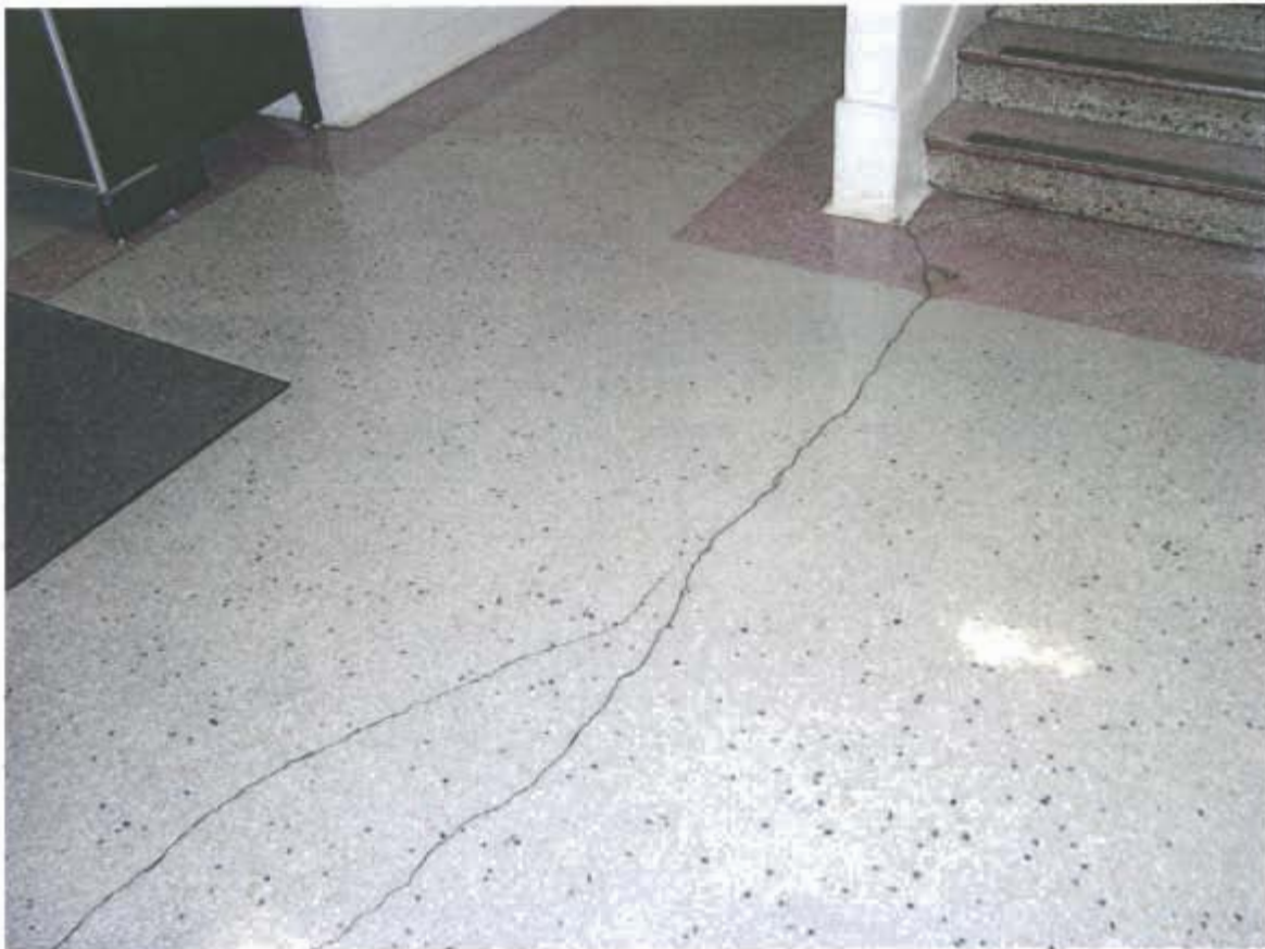
Photo #2: Random cracking in terrazzo floor at first floor near south stair.
