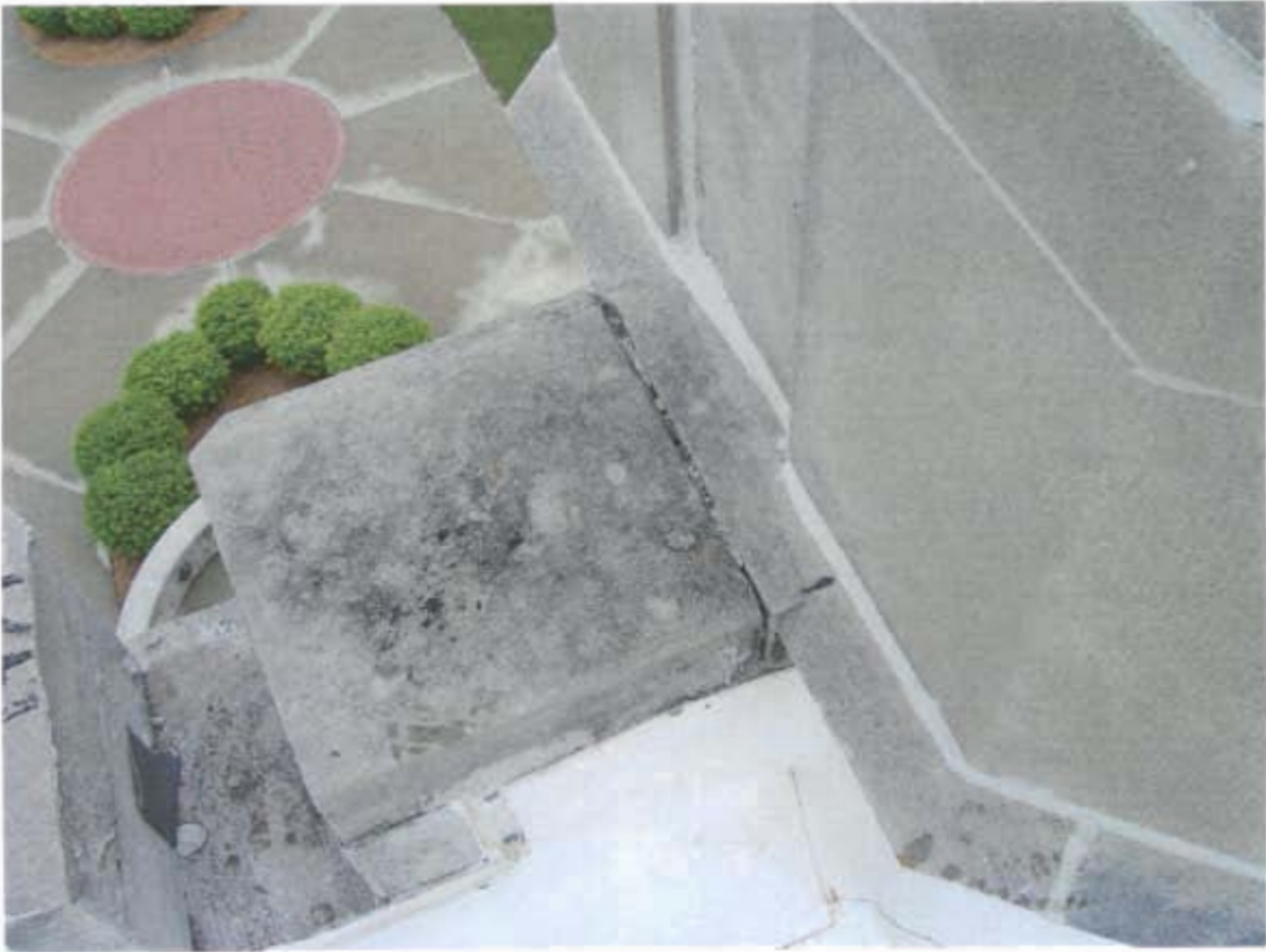
Photo #9: Failed caulk joint at stone cap between front entry towers.
