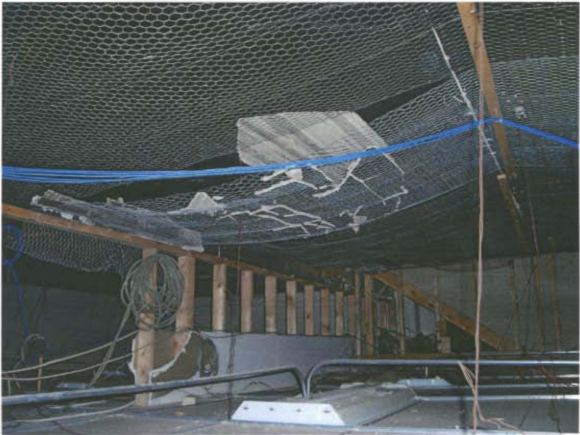
Photo #5: Falling plaster above first floor Library ceiling. Chicken wire installed to catch the plaster. Plaster was directly applied to concrete structure.
